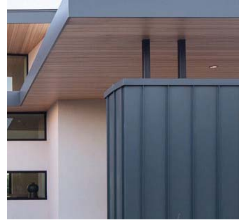
SIMILAR PALETTE OF STANDING SEAM METAL, STUCCO, BRAKE METAL, AND WOOD SOFFIT
